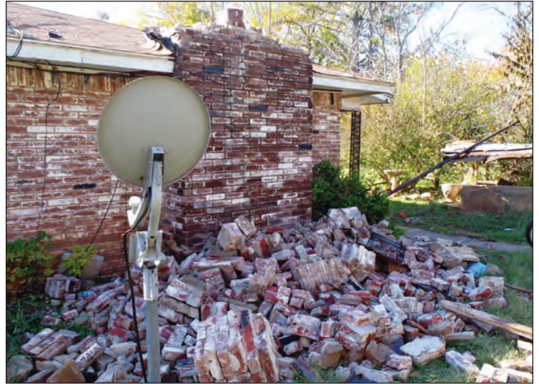
A government photo shows damage to a home in central Oklahoma from a magnitude 5.6 earthquake on November 6, 2011. Research conducted by the United States Geological Survey suggests the earthquake was induced by wastewater injection into deep disposal wells in the Wilzetta North field.
